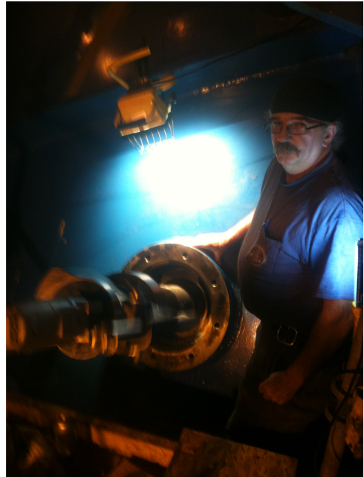
Pictured is IAM Local Lodge 818 President Charlie Mikels; he is performing field machining on a turbine draft tube at the New Martinsville, WV Hydro Electric Plant.
